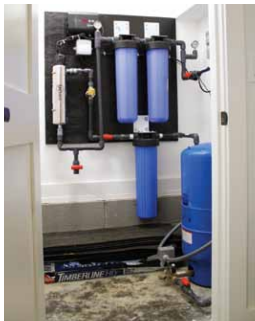
Top: Three 1,700-gal cisterns store the collected rainwater. Bottom: The rainwater is treated with sediment and carbon filters and UV to ensure safety and quality.
